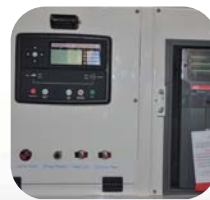
Control Panel & MCB
